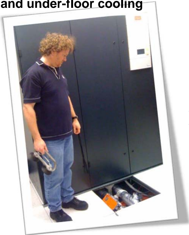
Andrew Munsie, Data Centre Manager, displaying the under-floor plumbing beneath a perimeter cooling Stulz CRAC unit
